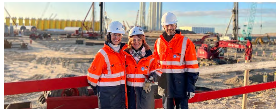
The sustainability team at Neste's renewable products refinery expansion project in Rotterdam
