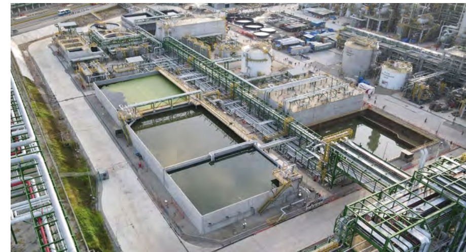
The Complex Wastewater Treatment Unit (CWWT) of the Long Son olefins plant in Vietnam started up in 2022 (Courtesy of Long Son Petrochemicals)
